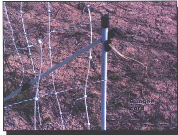
Figure 6—Bungee cords can be used to hold diagonal braces against corner posts.
